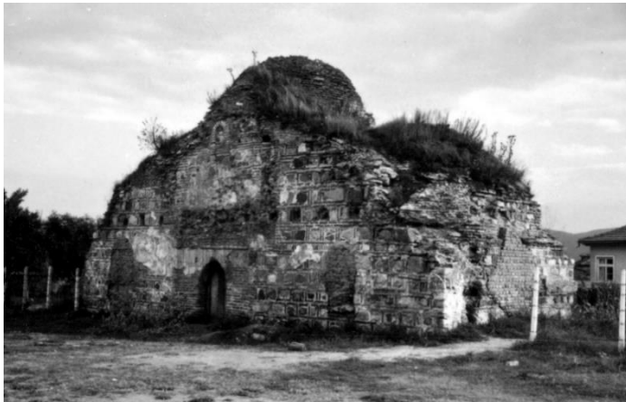
Figure 4. The zaviye building in Ihtiman. The general shape of the building is visible but the portico has apparently collapsed. The minaret is a later addition, from the time that the building was turned into a mosque. (Courtesy of Machiel Kiel Photo Archive, 1969).
